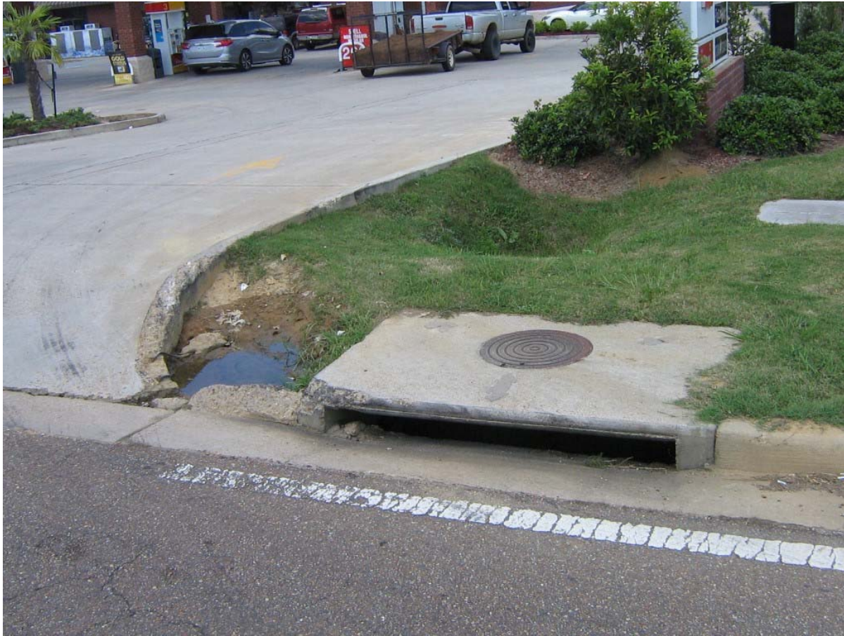
Above: Looking north at East Shell driveway from Gluckstadt Road – deficient turning radius.
