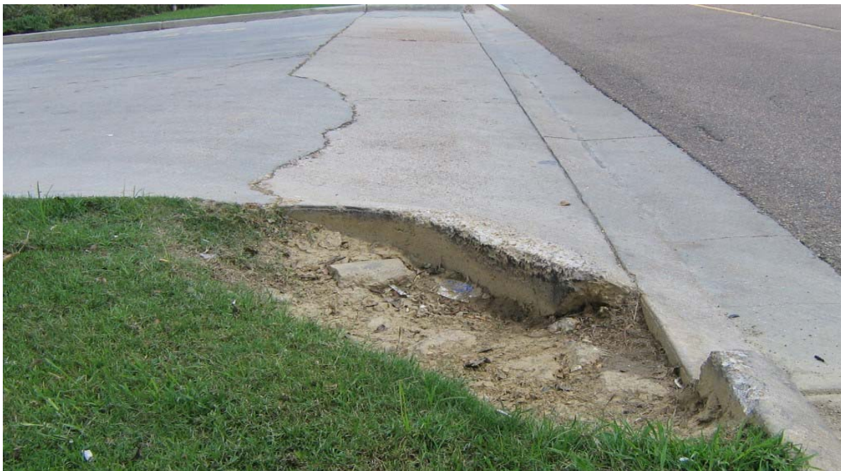
Below: Looking east at West Shell driveway from Gluckstadt Road – deficient turning radius.
