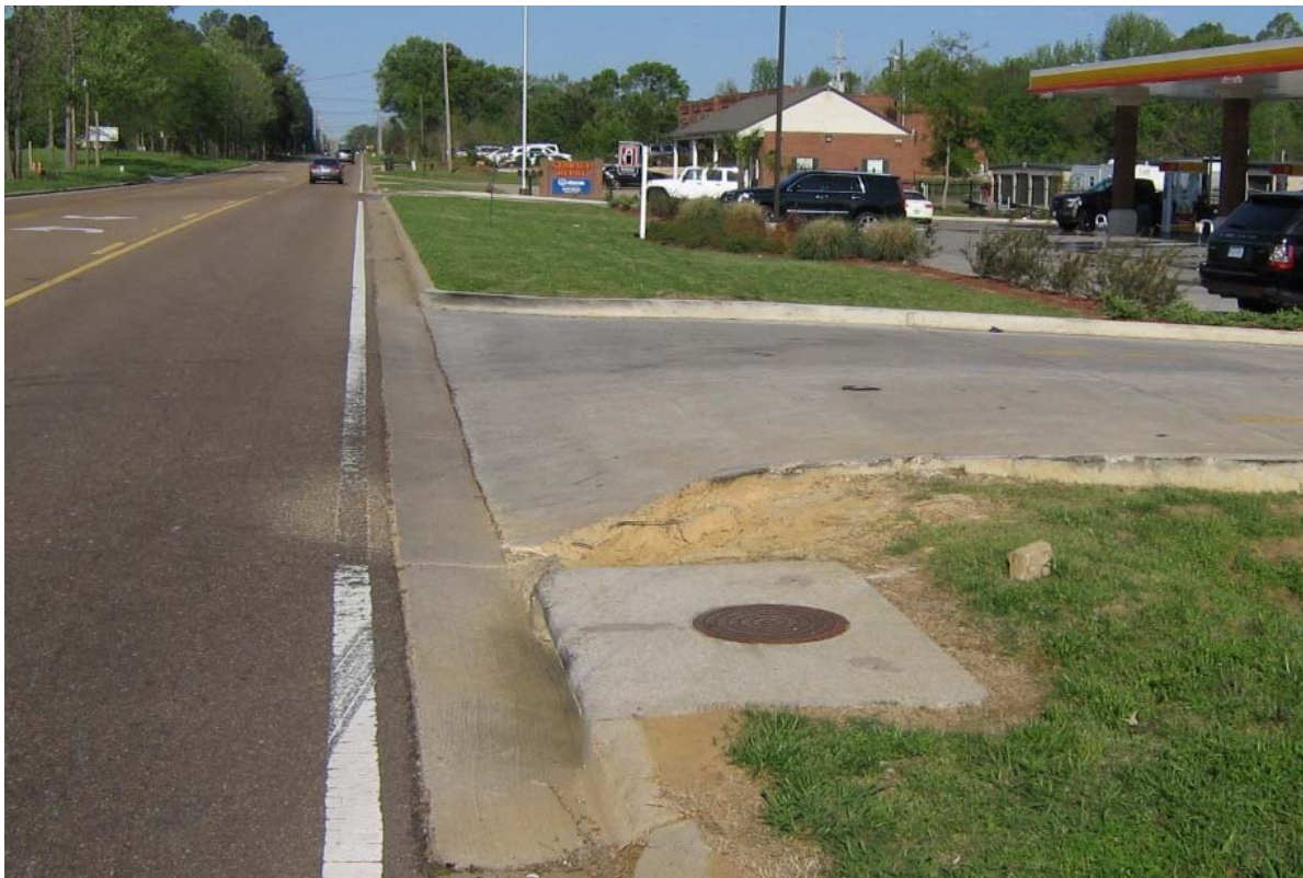
Driveway on Gluckstadt Road with insufficient turning radii.
